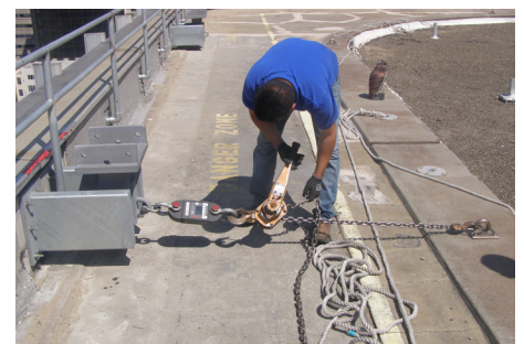
Direct pull test on an anchorage (right) by reacting off of a davit base (left).
