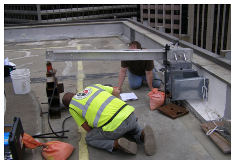
Load testing of a parapet-mounted davit base using a specialized test fixture.
