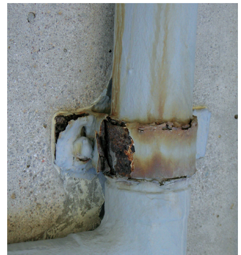
FIGURE 2 Galvanic corrosion of carbon steel clip angle connecting copper downspout to substrate (Photo by James Chiropolos of WJE).
