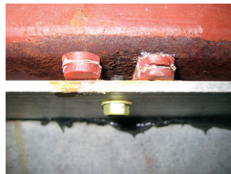
FIGURE 3 Galvanized steel fastener through aluminum kerf anchor (Photo by Fiona Aldous of WJE).
