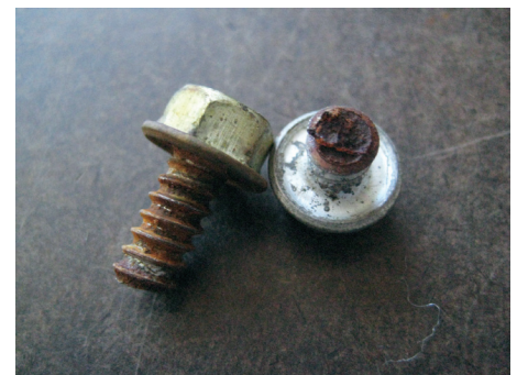
FIGURE 4 Fractured galvanized steel fasteners that were used with aluminum kerf anchors (Photo by Fiona Aldous of WJE).
