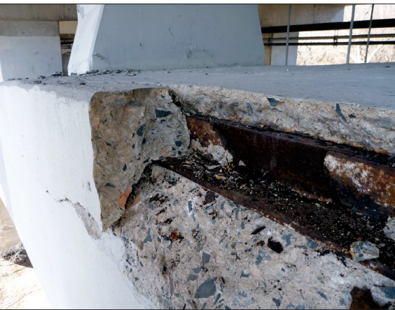
Fig. 7. Franklin Avenue Bridge, example of chloride-induced corrosion spalling along the arch-rib corner, 2012.
