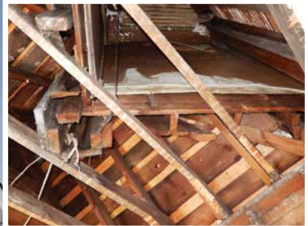
Figure 8. Partial view of framing above corner entrance added to the 1890s church in central Illinois. Note that the wall studs and corner framing was cut away without provision of any supplemental support.
