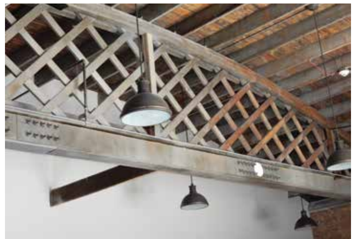
Figure 6. Partial view of lattice truss within the roof structure above the administration building.
