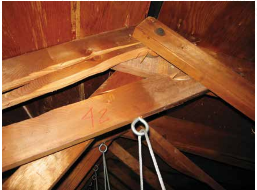
Figure 4. Fractured roof truss members at split-ring connectors attributed to high perpendicular-to-grain loading of members.
