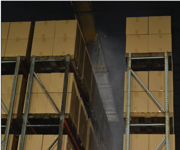
The use of K14 sprinklers was initially discounted given the recent controversy regarding the adequacy of K14 sprinklers to protect rack arrays of Group A plastic beneath a 40-foot ceiling. However, the extensive legacy use of the K14 sprinkler prompted the exploration of its performance in Phase 4. Photo: Wiss, Janney, Elstner Associates, Inc.
