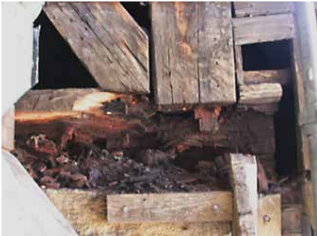
Figure 1. Advance decay in a timber framed bell tower (left) - (Crowe Photo).
