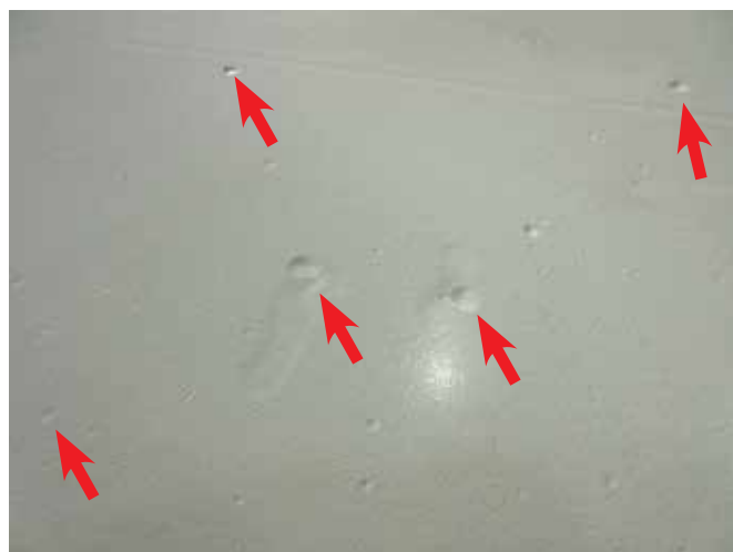
Fig. 1: Blisters in an airport hangar floor coating (larger ones shown with red arrows)
