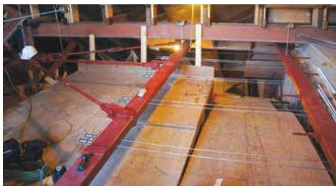
Figure 4. View of nitinol fuses as installed in the attic of Sherith Israel
