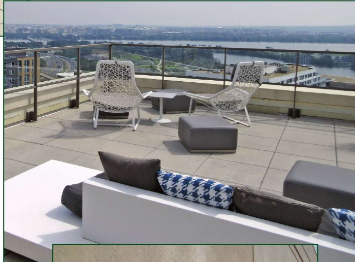
Figure 4. Consideration should be given to existing parapet heights and code requirements for guardrails. Existing parapets or guardrails may require modification to meet code requirements.
