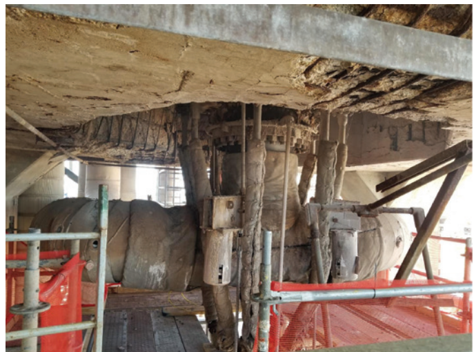
Figure 2. View of octagonal penetration in upper deck and piping associated with the catalytic reformer.
