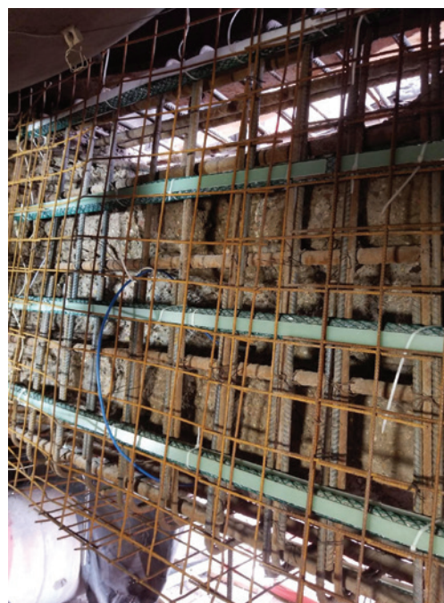
Figure 7. Welded wire reinforcing, galvanic anodes (arrows), and concrete maturity meter in repair area.
