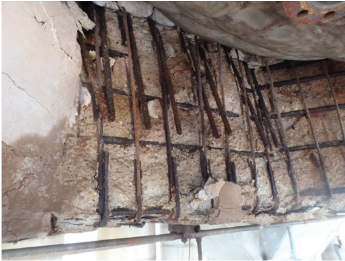
Figure 3. Spalled concrete with exposed reinforcing on the sides of the octagonal penetration in the upper deck (fractured stirrups are visible).
