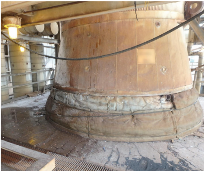
Figure 4. Widespread cracking on top of upper deck, typically emanating radially from the catalytic reformer.
