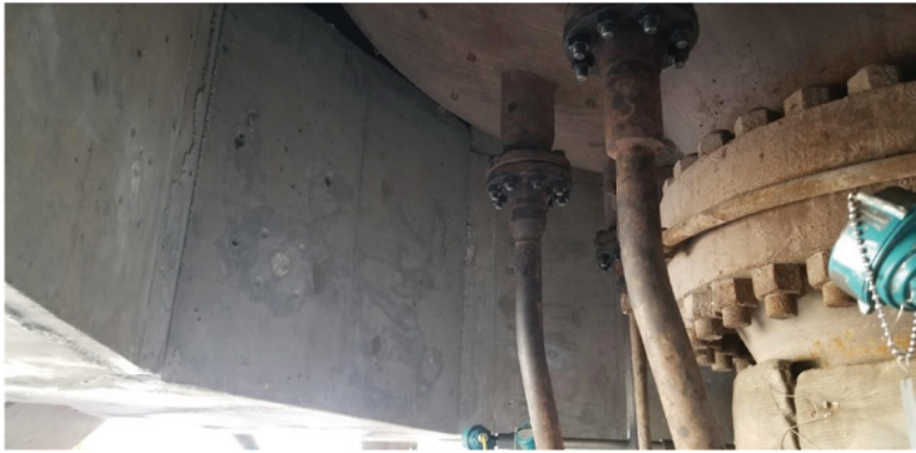
Figure 8. Completed repair on the sides of the octagonal penetration in the upper deck.
